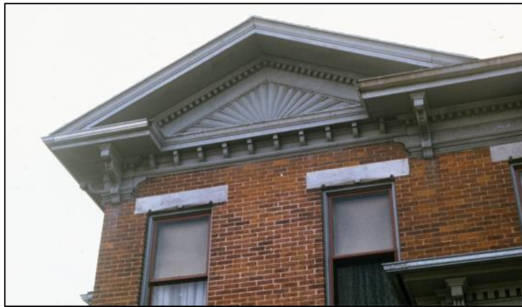
Looking up we see the same arrangement of forms in the roof cornice. Photo taken by Dr. Les Crocker, 2020.
