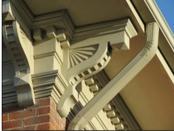
Bracket detail on a corner of the house. Photo taken by Anita Taylor Doering, 2019.
