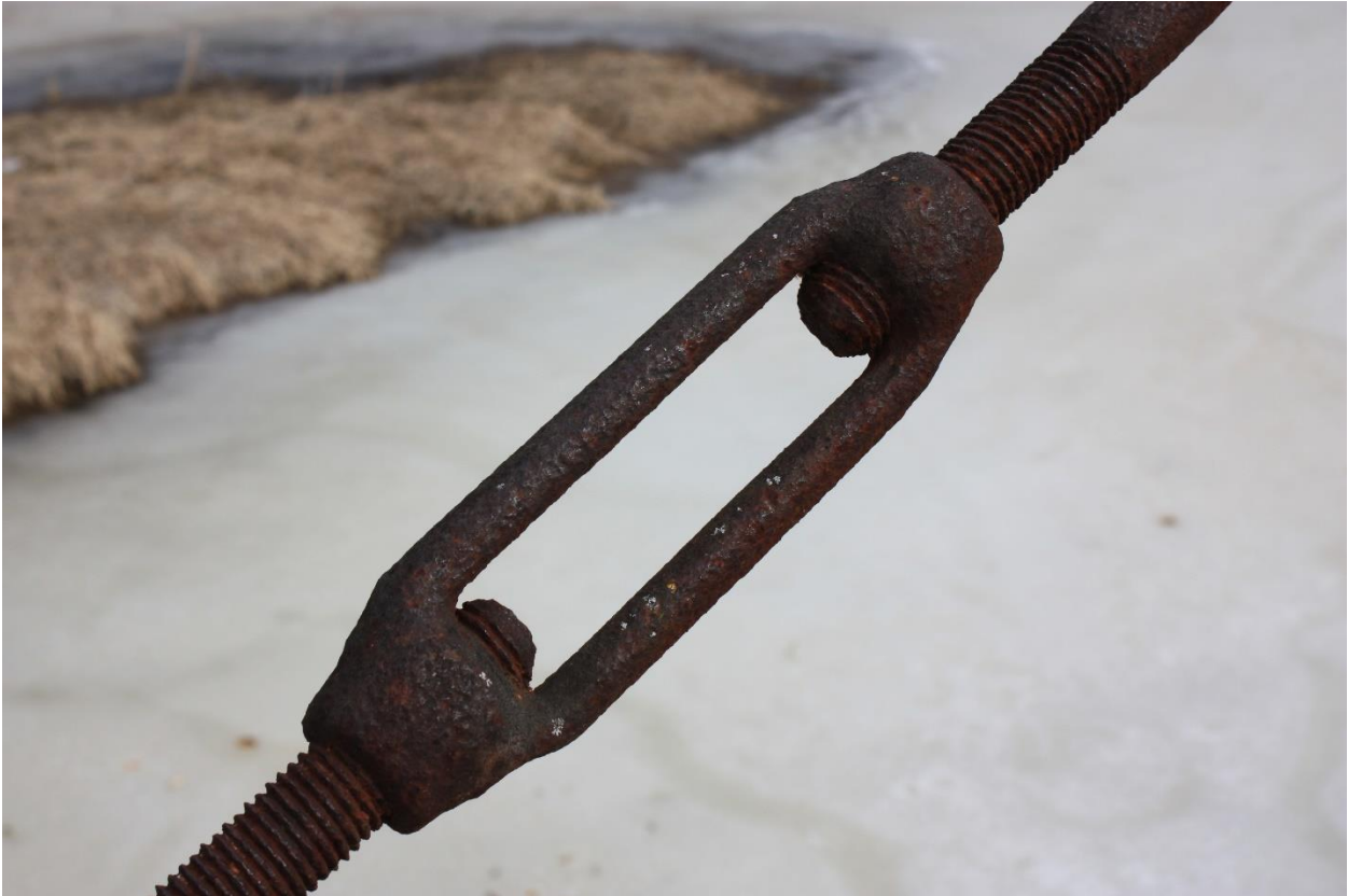
Adjustable turnbuckle on a diagonal support
